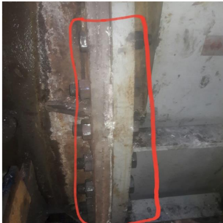
Figure 1. Leak area that is tried to be removed by welding
