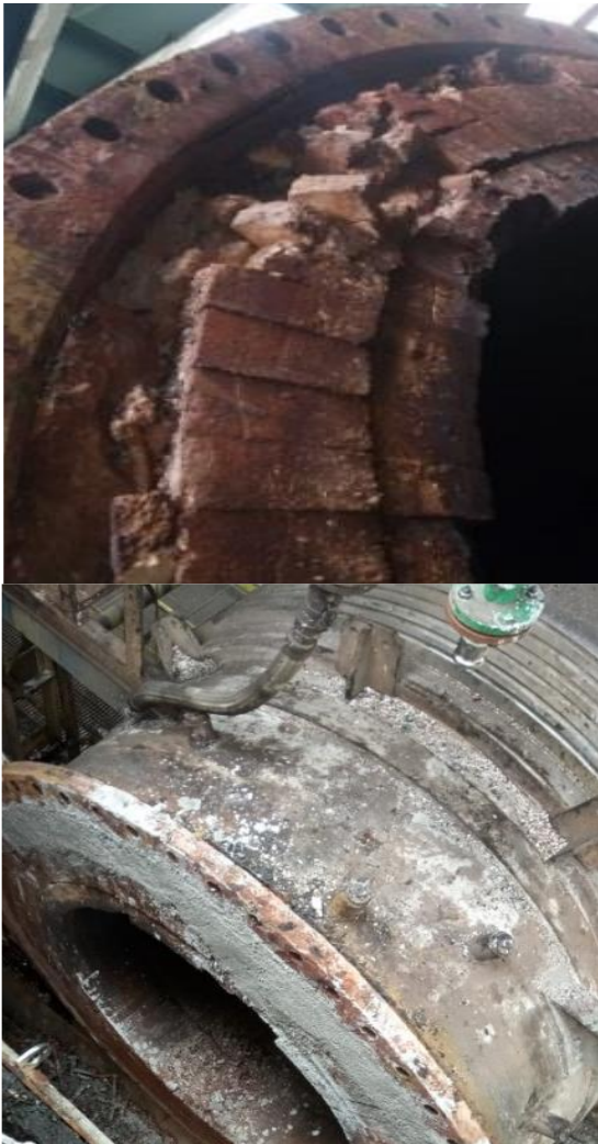
Figure 5: Wear of refractory materials in flanges areas
