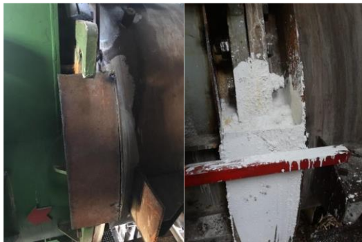
Figure 8: Flange areas of valves are molded with pattern and concrete is poured into pattern
