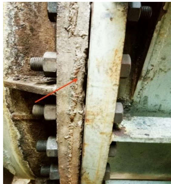
Figure 4: Leakage from the flange connection areas of the valves
